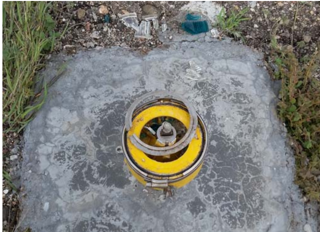
Figure 2: The broken runway light
