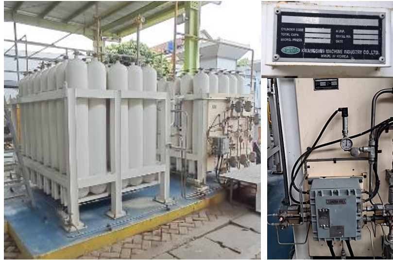
Gambar 27. Storage tank gas CNG
